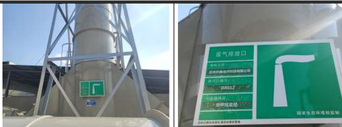
DA012 废气排气筒
